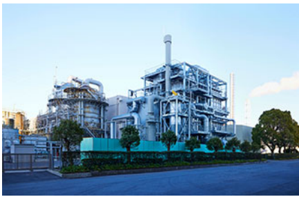
Biomass boiler (Chita Distillery)
